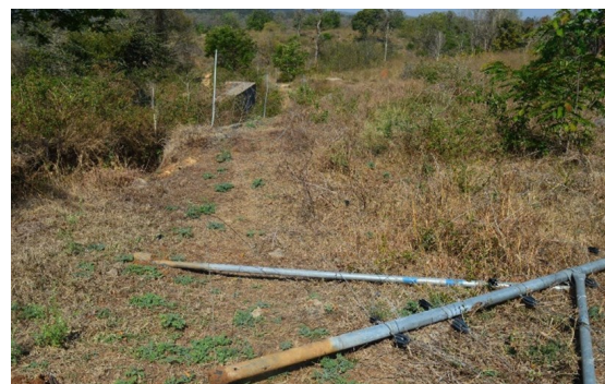
Figure 7. Breakage on Solar Fence
